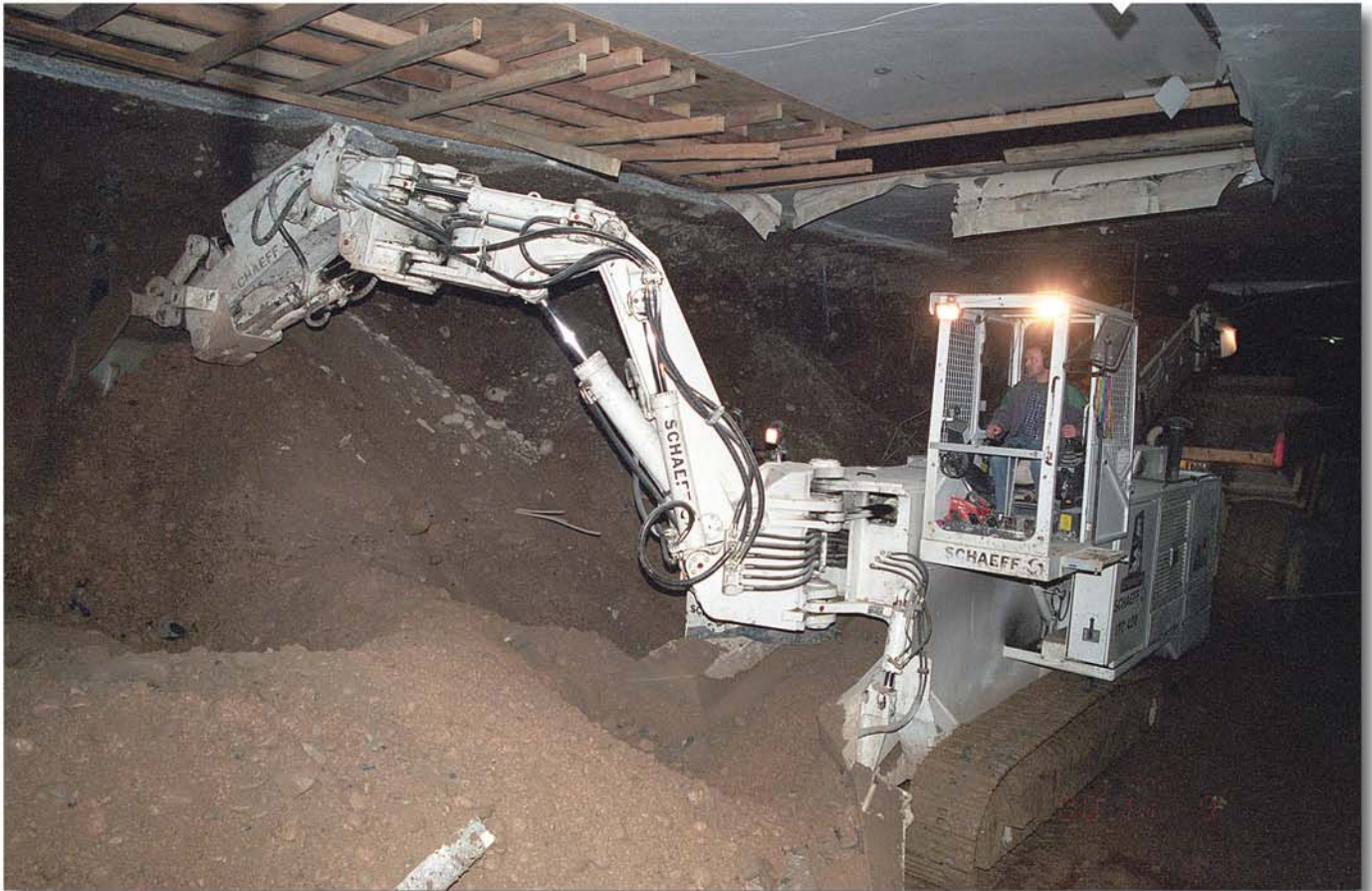
The Tunnel heading and loading machine Schaeff model ITC 420 powerful demolition in a cut and cover tunnel
