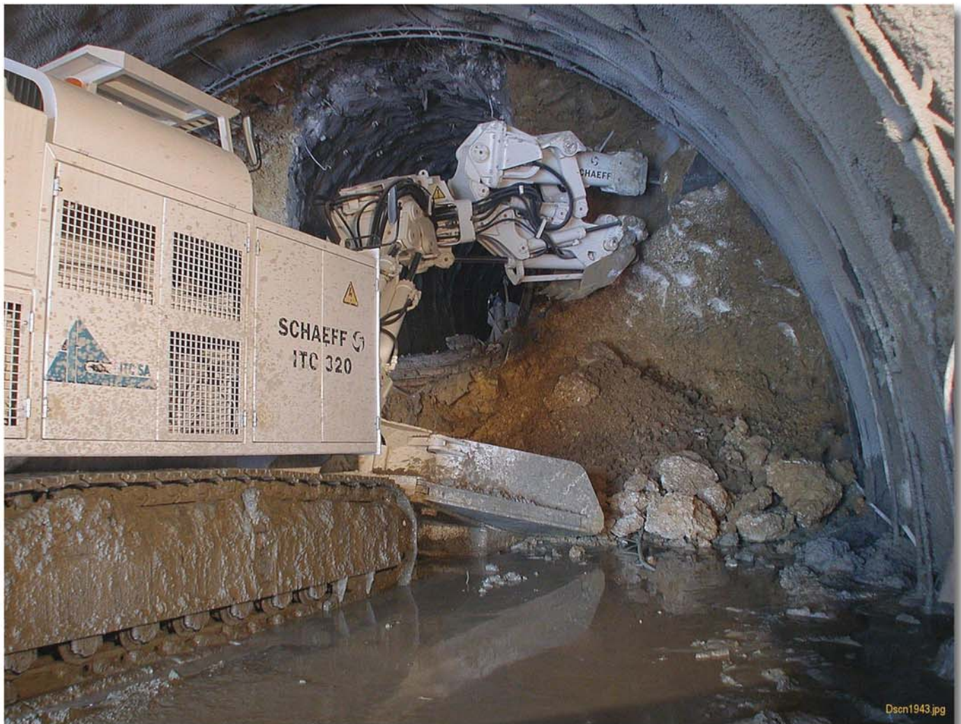
Fig 1 : Hammer heading the east portal. Tunnel heading and loading machine Schaeff type ITC 320
