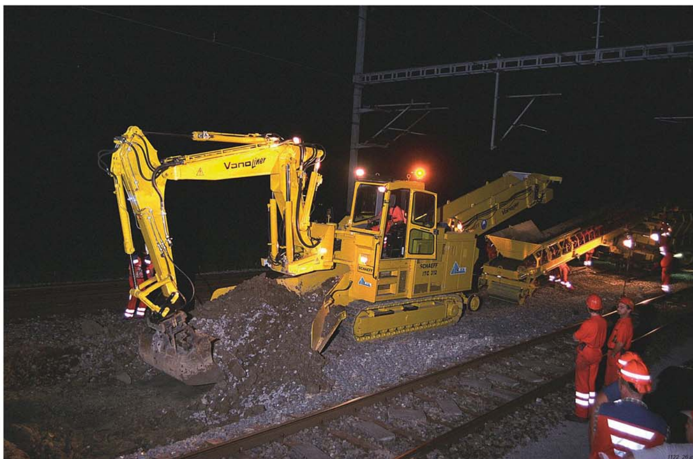
Pict. 1: Ballast loading machine Schaeff type ITC 312 excavating within the close vicinity of station AU (ZH)
