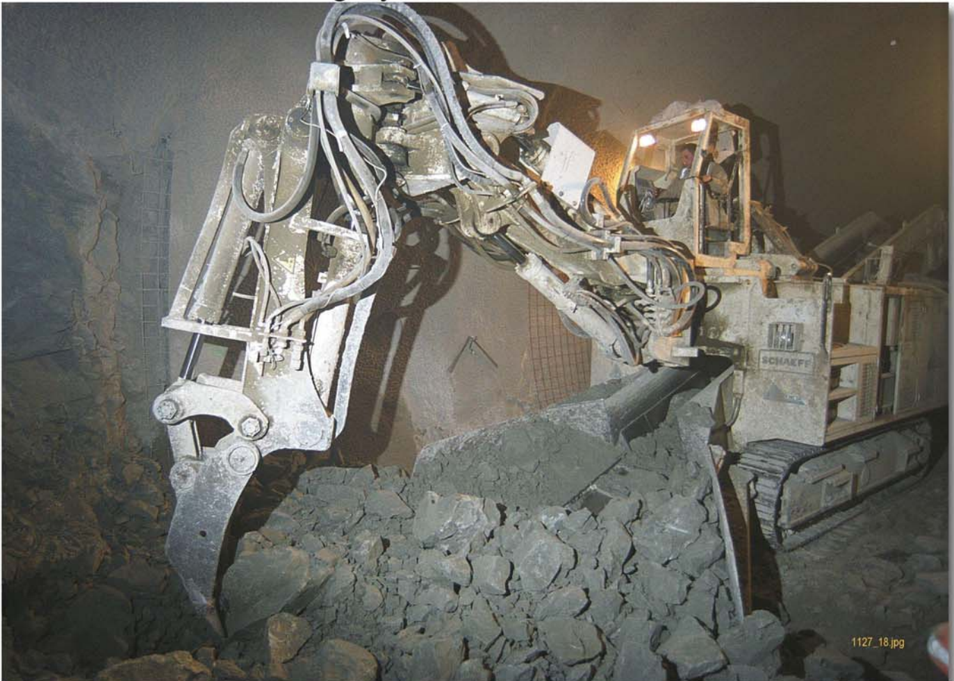
Fig. 1: Schaeff Tunnel Heading & Loading Machine Type ITC 312H1 in conventional tunnelling in the second tube tunnel
