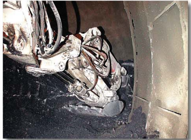
7: ITC 420 in South Heading, Loosening
