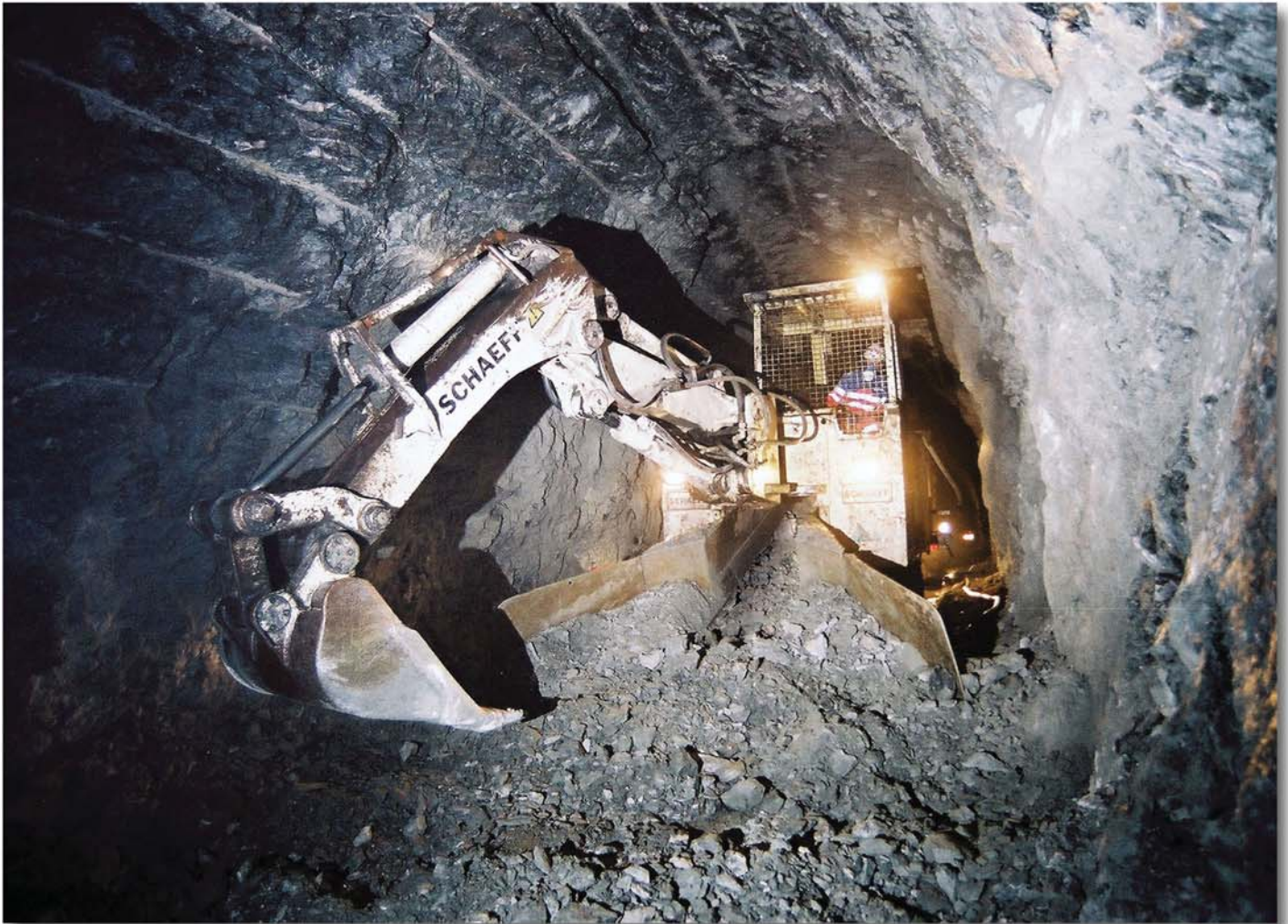
Picture 1: The mucking machine Schaeff model ITC 312 H3 at work in Hhydro Power Plant Follafoss
