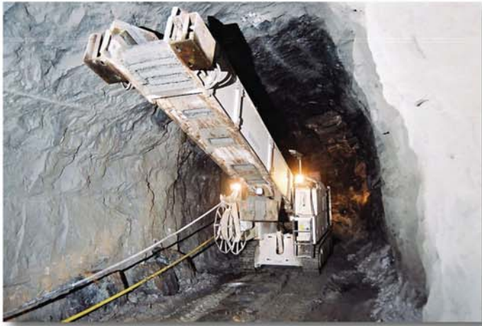
Picture 4: Rear view of the mucking machine ITC 312 H3 with cable reel for the electric drive
