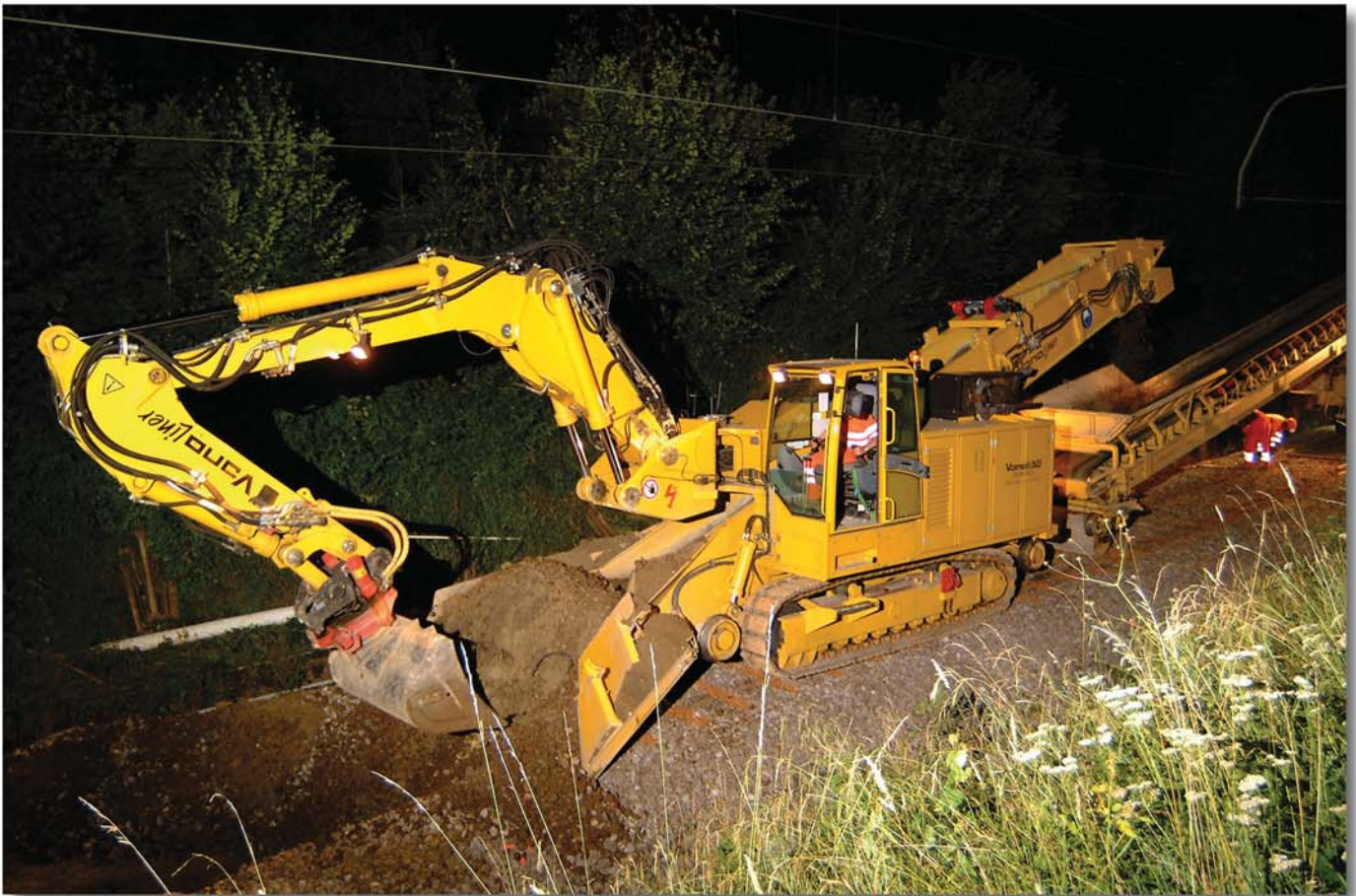
The ballast loading machine Schaeff model ITC 312 Vanoliner with jointed boom in loading position
