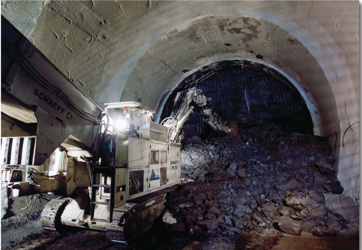
The Tunnel Heading Machine Schaeff model ITC 312 N1 in excavation position under the concrete prevaults
