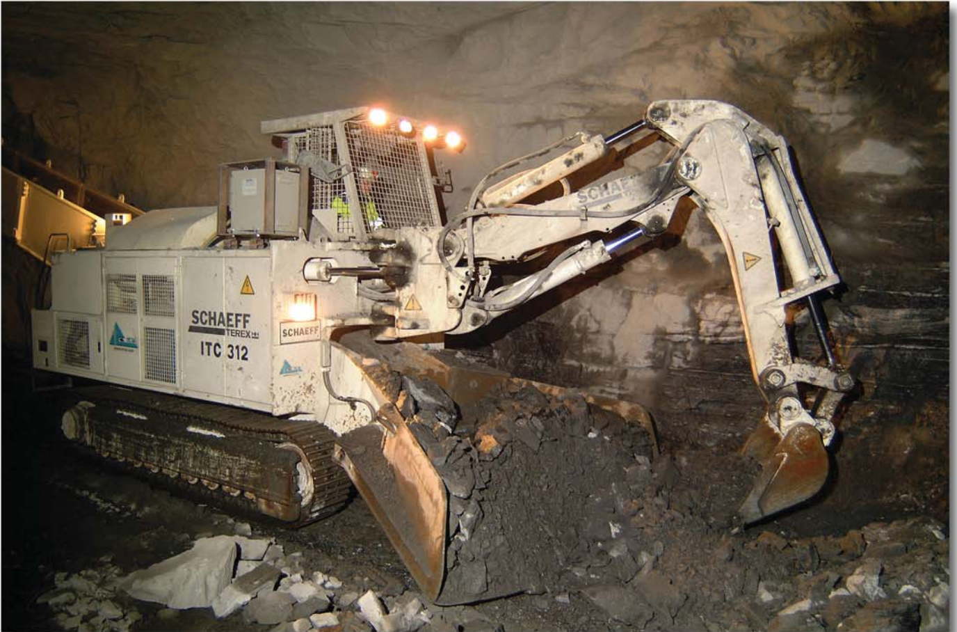
The loading machine Schaeff model ITC 312 by cleaning the invert in 1:8 incline
