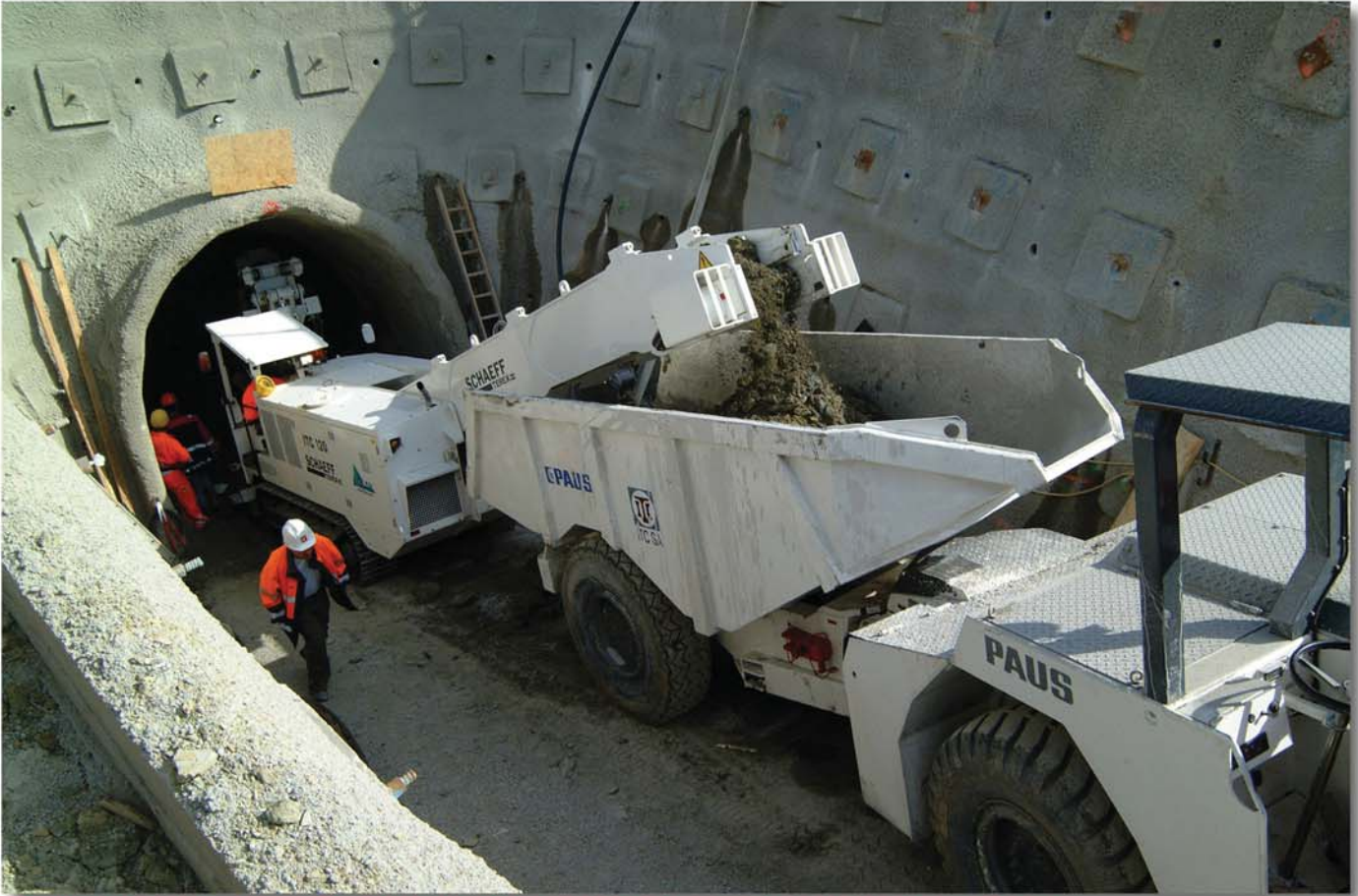
The Tunnel Heading Machine Schaeff model ITC 120 loading onto a dump truck Paus model ITC 8000
