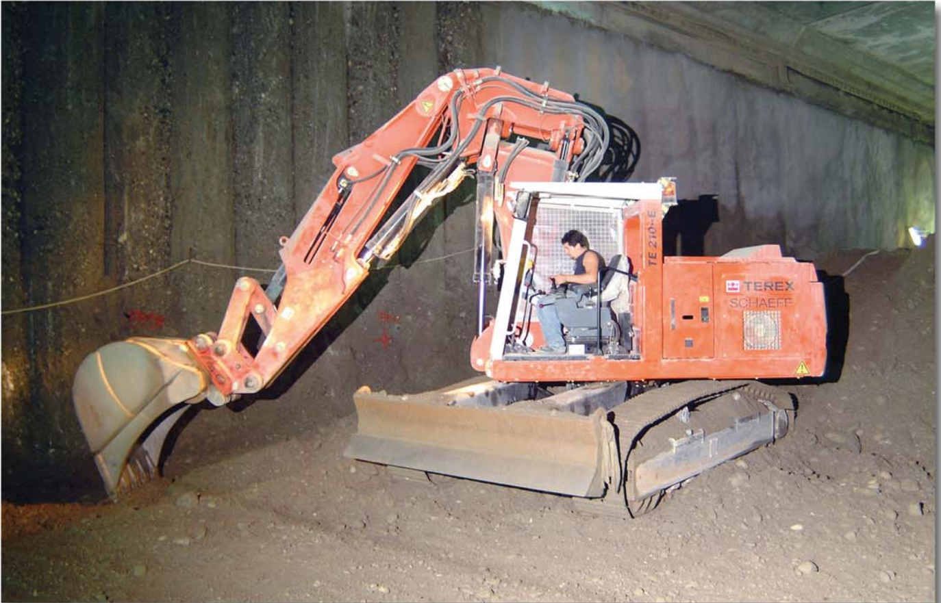
The electric Tunnel excavator model TE 210 E excavating the invert between the grouted piles
