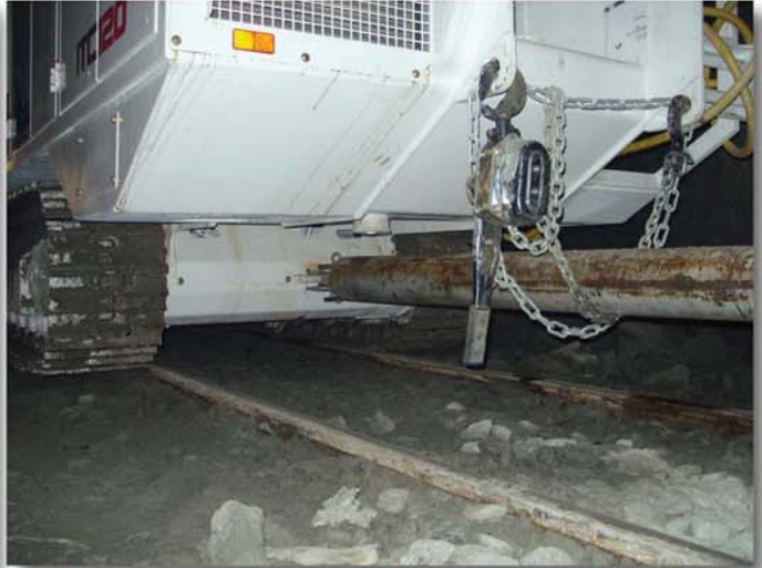
Rigid link between loading machine and backup, both on 900 mm rail gauge
