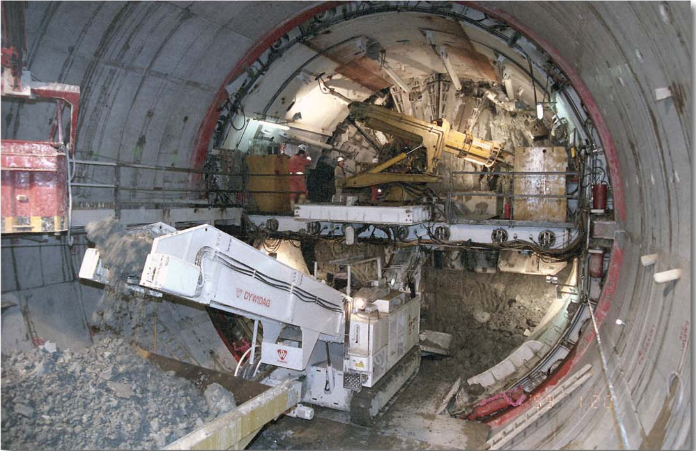
The Tunnel heading and loading machine Schaeff model ITC 3i2 in the shield
