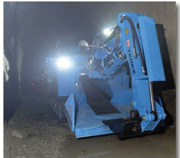
The Superloader in travelling position in tunnel
